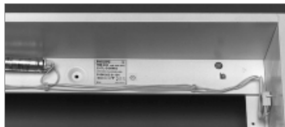
Fig. 140 Solid-core wire inside a luminaire for fluorescent lamps. White wires are used where the wiring is visible from below.
